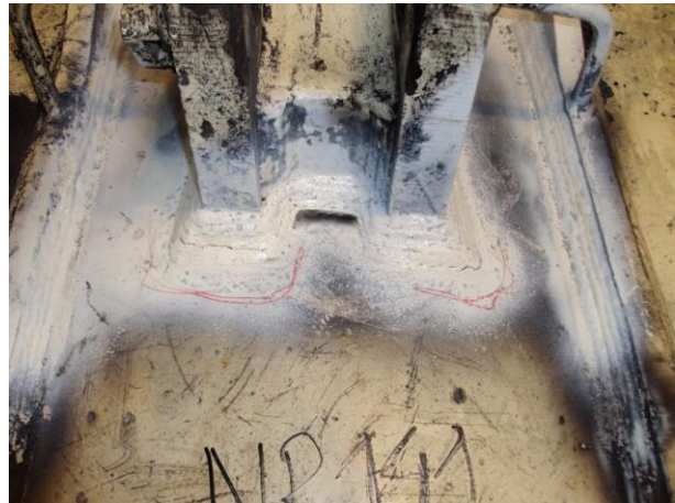
Fig. 2. Damaged welds in the gob shield of roof support No. 135[12]
