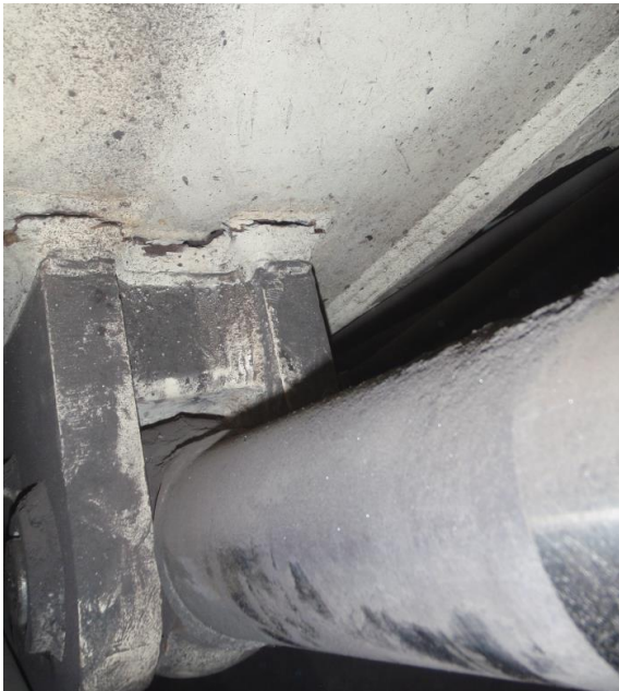
Fig. 1. Damages to the welds connecting the lifting eye system of the tilt cylinder with a gob shield sheathing sheet [12]
