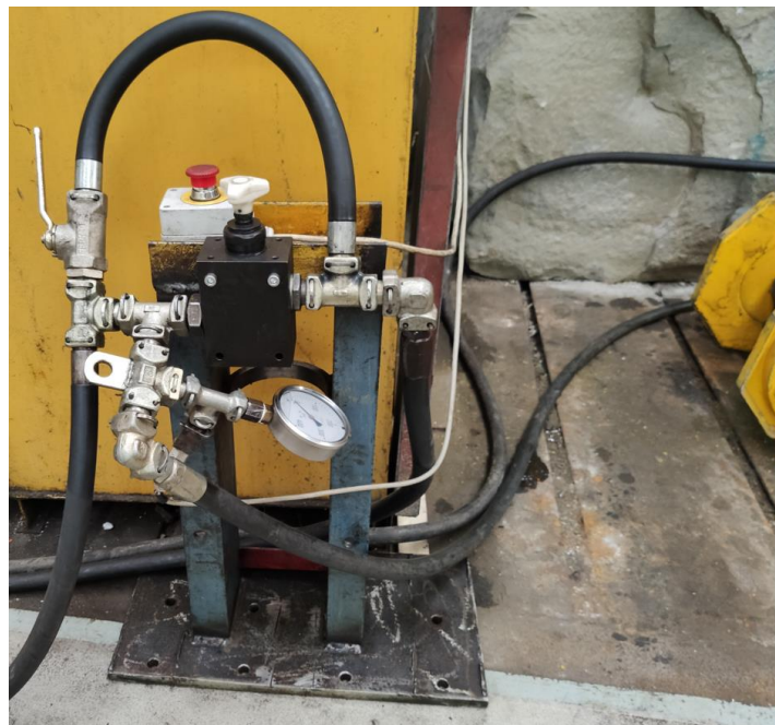
Fig. 4. Hydraulic control unit
